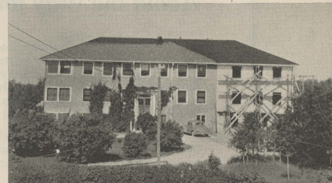
Vita General Hospital, Vita, Man., showing new addition in process of construction, 1940. Dr. H. V. Waldon has been Superintendent of this Hospital since 1927
